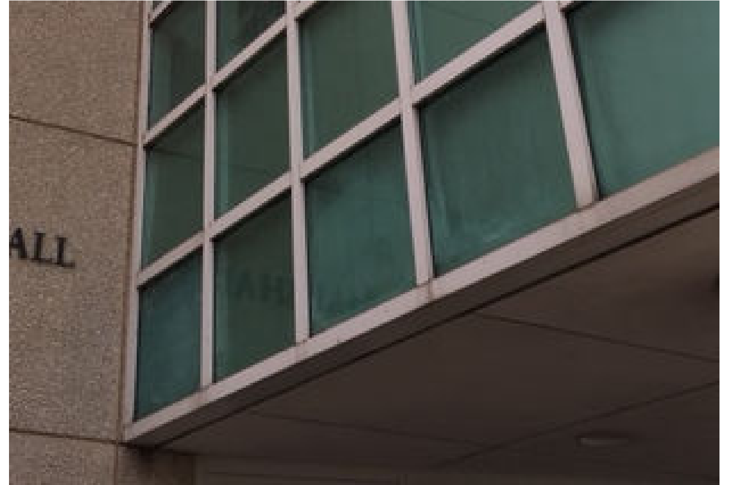
Dust and Debris Infiltration
