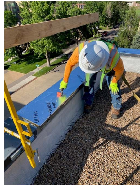
Parapet cap removed, surface coated with adhesive primer, tie-in flashing installed, and parapet cap replaced
