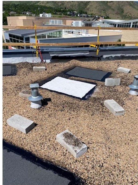
White + Black Roof Membranes
