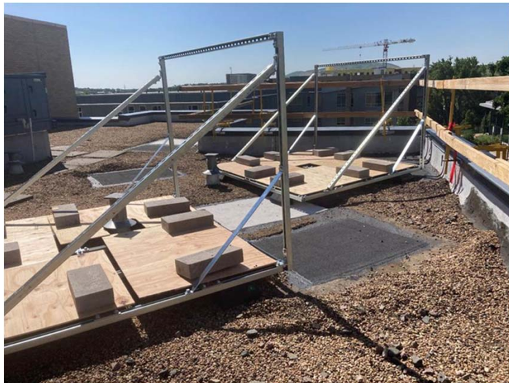
Vertical Reflective Surface Mounting Frames on Unistrut Sleds
