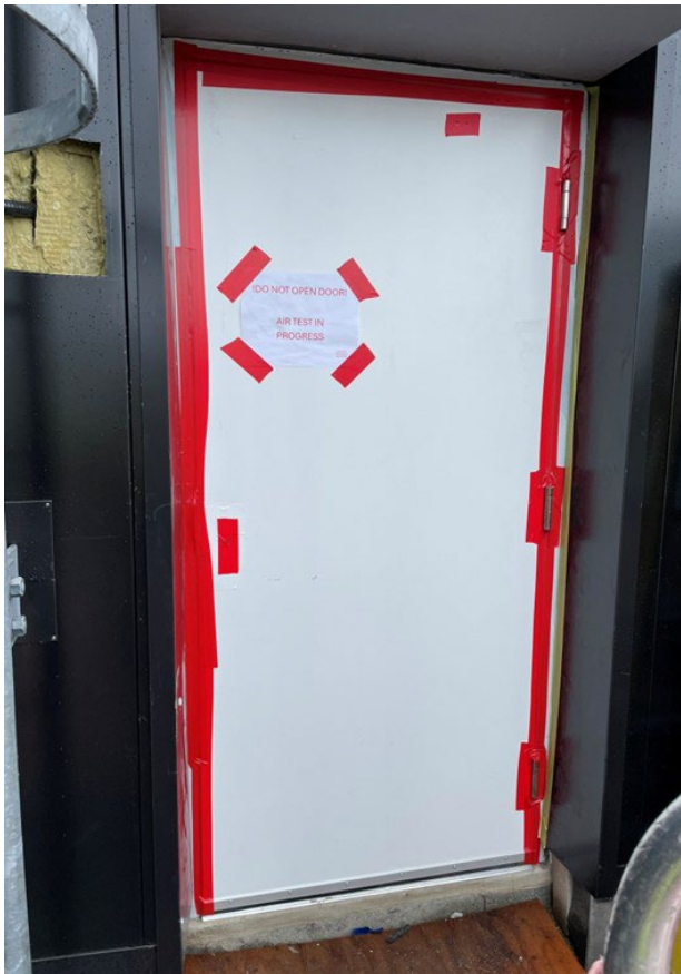
Elevator overrun roof door masked shut due to missing door hardware and gasket.
