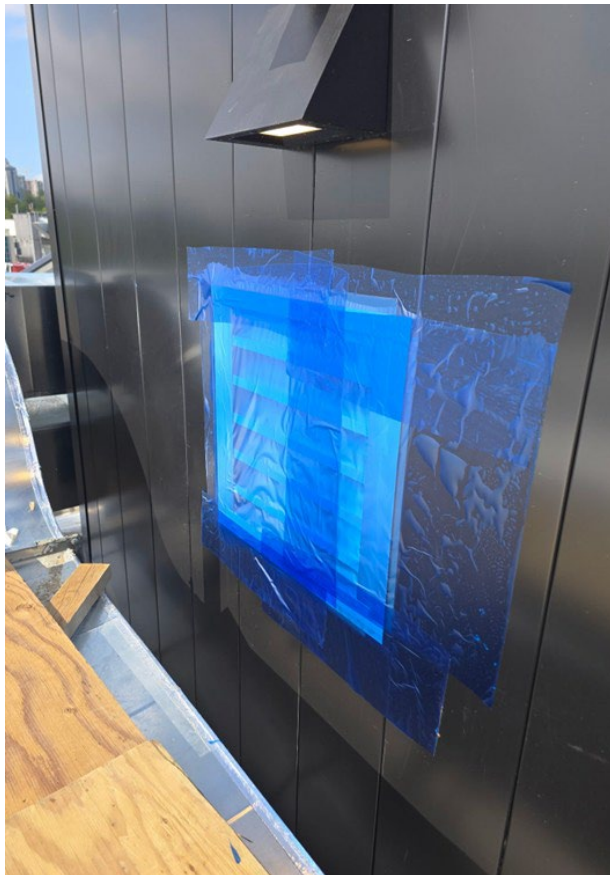
Elevator overrun exhaust masked shut from outside, done last to prevent overheating.
