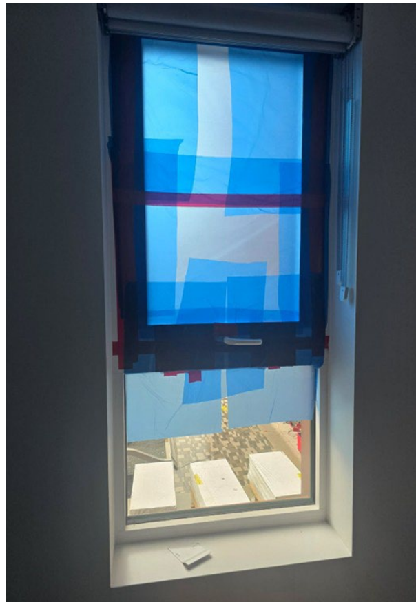
Unit 246 window masked shut due to hardware not latching.
