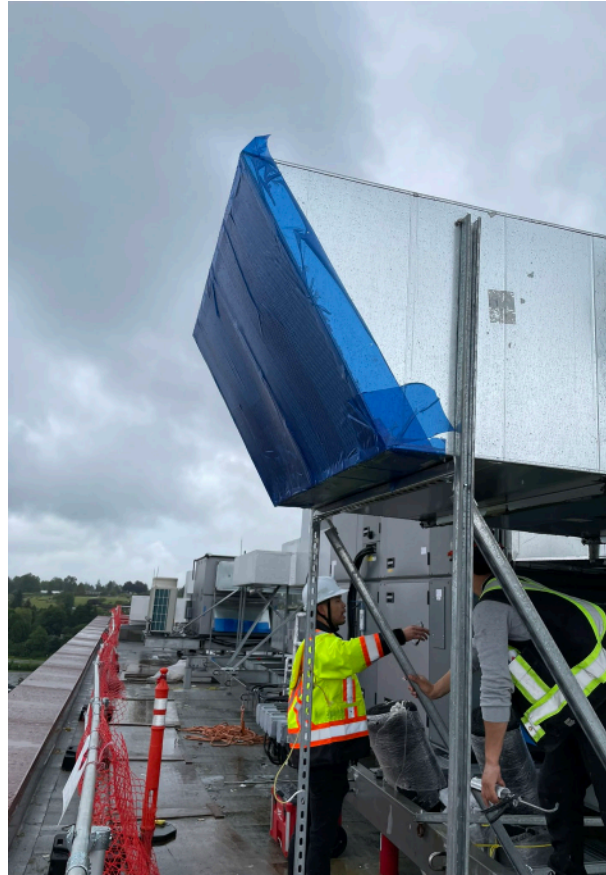
Air Handling units sealed.
