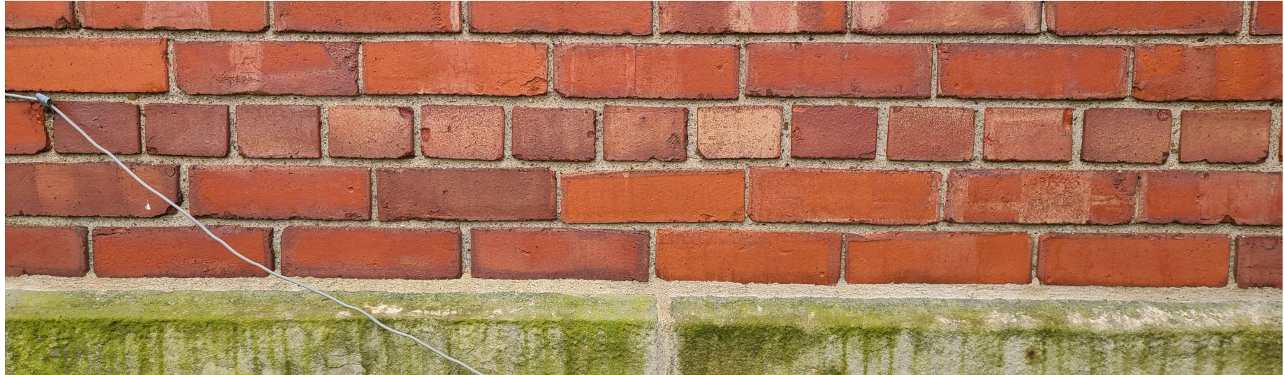
No Flashing & Weeps
