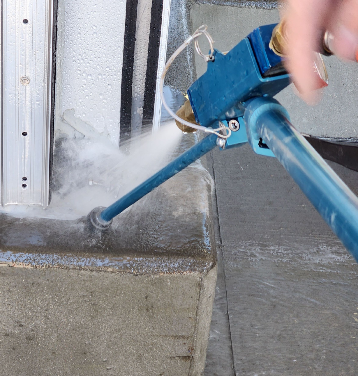
In-Place Water Spray Testing
